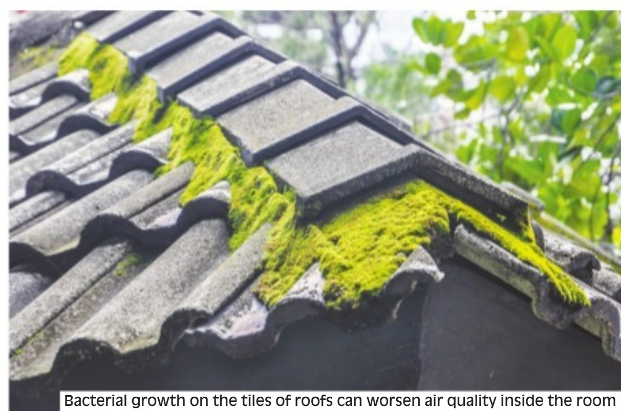
Bacterial growth on the tiles of roofs can worsen air quality inside the room
